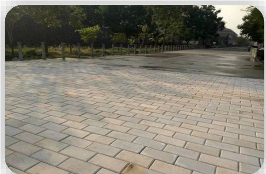
APP BRICKS – DIVIDER ON HIGHWAYS
